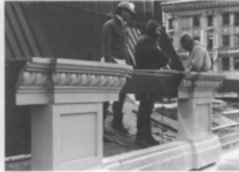
Illus. 18. Substitute materials must be properly installed to allow for expansion, contraction, and structural security. The new balustrade (a polymer concrete modified with glass fibers) at Carnegie Hall, New York City, was installed with steel structural supports to allow window-washing equipment to be suspended securely. In addition, the formulation of this predominantly epoxy material allowed for the natural expansion and contraction within the predesignated joints. Photo: Courtesy of MJM Studios.
