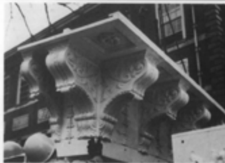
A fiberglass cornice for the reconstruction of an 18th-century wooden clockcase is being lifted in pre-fabricated sections. The level of detail is intricate and of high quality. Photo: Courtesy of Independence National Historical Park.
