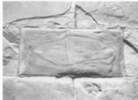
Illus. 19. When the physical properties are not matched, particularly thermal expansion and contraction properties, great damage can occur. In this case, an extremely rigid epoxy replacement unit was installed in a historic masonry wall. Because the epoxy was not modified with fillers, it did not expand or contract systematically with the natural stones in the wall surrounding it. Pressure built up resulting in a vertical crack at the center of the unit, and spalled edges to every historic stone that was adjacent to the rigid unit. Photo: Walter M. Sontheimer.
