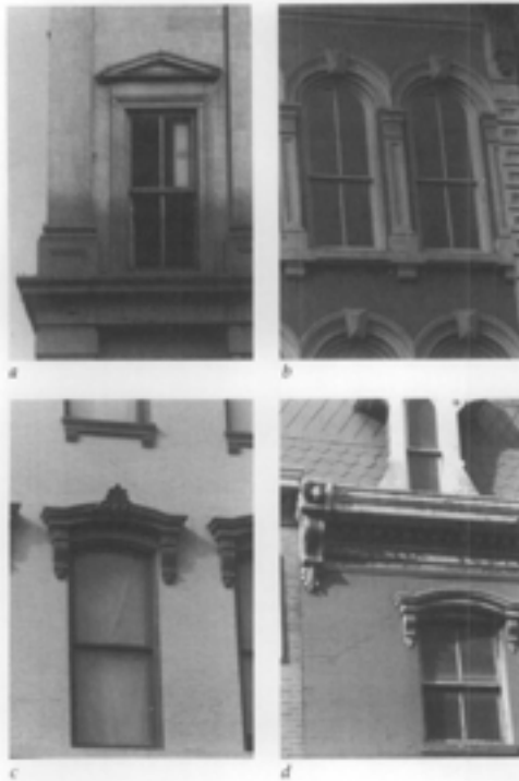
Illus. 5. The four historic examples of various window hoods shown are: (a) stone; (b) cast stone; (c) cast-iron; and (d) sheet metal. The criteria for selecting substitute materials today (availability, quality, delivery dates, cost) are not much different from the past. Photo: Sharon C. Park, AIA.
