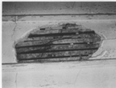
Fig. 13. This beaded ceiling in one of the bedrooms of the 1847 Lockwood House, Harpers Ferry, West Virginia, is missing portions of plaster due to broken keys. This is attributable, in part, to deterioration of the wood lath. Photo: Kaye Ellen Simonson.
