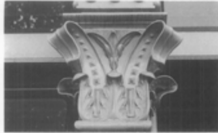
Close-up detail showing the crisp casting in aluminum of this 19th-century replica columns and capital for a storefront. Photo: Sharon C. Park, AIA.
