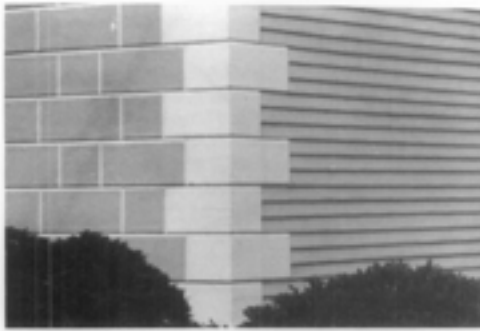
Illus. 1. An early 18th-century technique for imitating carved or quarried stone was the use of sand-impregnated paint applied to wood. The facade stones and quoins are of wood. The Lindens (1754), Washington, D.C. Photo: Sharon C. Park, AIA.
