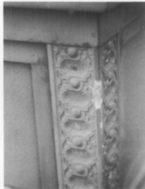
Illus. 20. Long-term performance can be affected by where the substitute material is located. In this case, fiberglass was used as part of a storefront at street level. Due to the brittle nature of the material and the frequency of impact likely to occur at this location, an unsightly chip has resulted. Photo: Sharon C. Park, AIA.
