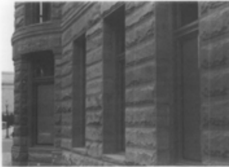
Illus. 16. The good quality substitute materials shown here do match the historic sandstone in color, texture, tooling and surface details. Dry-tamp cast stone was used to match the red sandstone that was no longer available. The reconstructed first floor incorporated both historic and substitute materials. Sufficient molds were made to avoid the problem of detecting the substitutes by their uniformity. Photo: Sharon C. Park, AIA.
