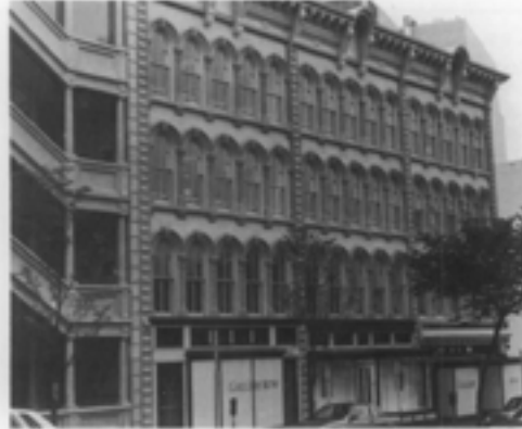
Illus. 22. A fiber reinforced polymer (fiberglass) cornice and precast concrete elements replaced deteriorated features on the 19th-century exterior. Photo: Sharon C. Park, AIA.
