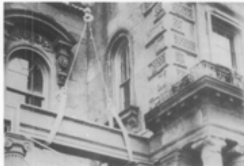
Illus. 9. Simple solutions should not be overlooked when materials are no longer available. In the case of the Morse-Libby Mansion (1859), Portland, ME, the deteriorated brownstone perch beam was replaced with a carved wooden beam painted with sand impregnated paint. Photo: Stephen Sewall.
