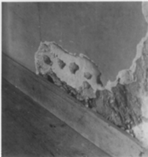
Fig. 4. The builders of this mid-18th century house installed the baseboard moulding first, then applied a mud and horse hair plaster (called paling) to the masonry wall. Lime was used for the finish plaster. Also shown are the backing marks which prepared the wall for a subsequent layer of plaster. Photo: Kay Wecks.
