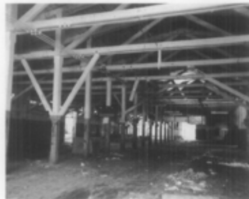
Figure 2. The interiors of mills and industrial buildings frequently are open, unadorned spaces with exposed structural elements. While the new uses to which this space could be put are many—retail, residential, or office—the generous floor-to-ceiling height and exposed truss system are important character-defining features and should be retained in the process of rehabilitation.
