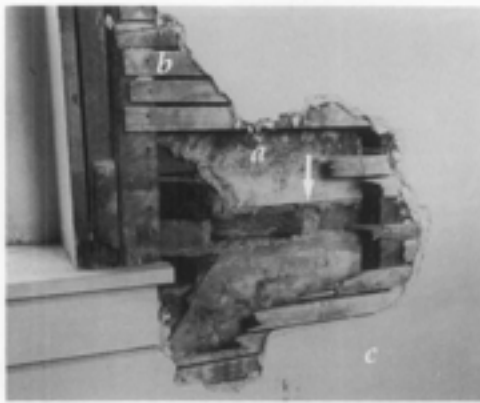
Fig. 2. A hole in the wall of a 1760s Custom House in Chestertown, Maryland illustrates the evolution of the room. (a) The original plaster was applied directly to an exterior masonry wall and the chair rail (missing here, see arrow) was in place before the wet plaster was applied to the wall. Sometime later when the interior was modified, the masonry was furred out. Machine-sawn wood lath (b) was nailed to the furring strips and (c) new three-coat plaster was applied. Photo: Maryland Historical Trust.
