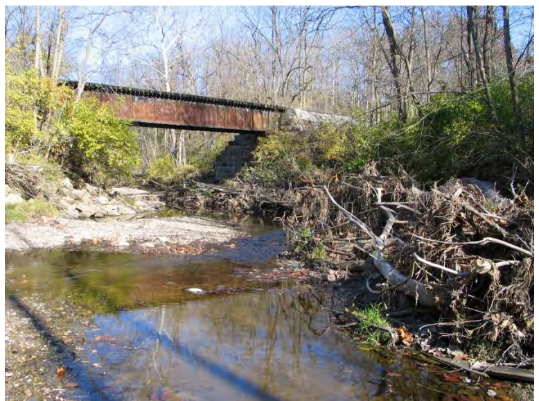
Exposed existing trunk sewer with railroad bridge in background & flood damage
