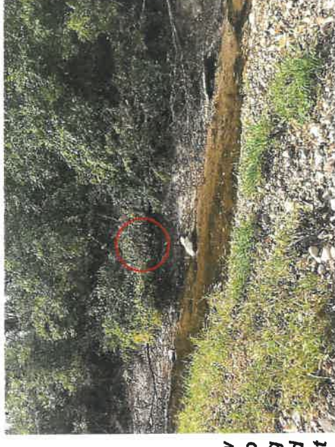
Staking for new alignment eroded into Farm Creek during Summer 2020 flood event
