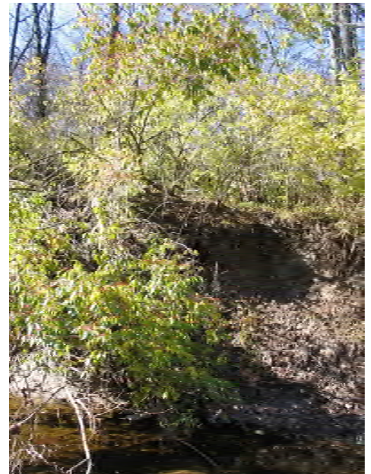
11 ft. bank ht. w/ new trunk sewer marker stake above rt
